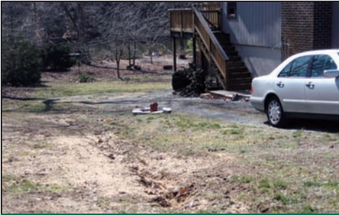
Improper yard maintenance causes erosion.
